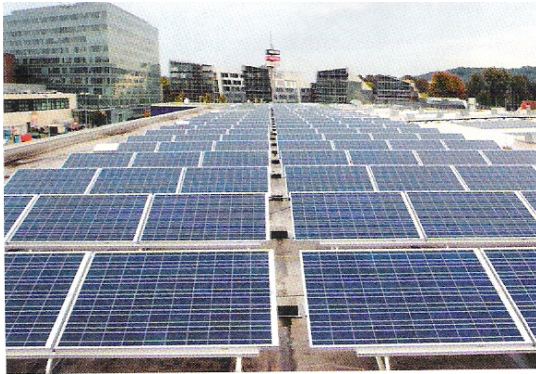
Figure: PV modules mounted on an open rack construction on a flat roof
